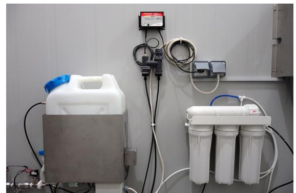
Integrated water treatment systems
